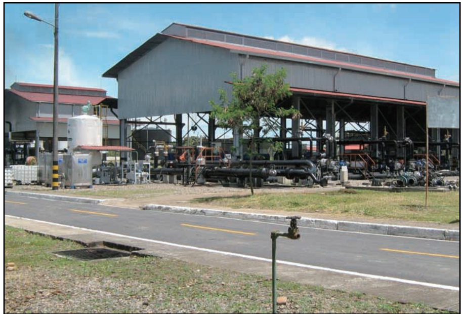
An ExtremePower™ Flow Improver injection system sits in the lush landscape of Colombia.
